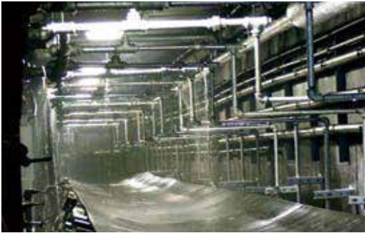
Conveyor gallery Washdown System
