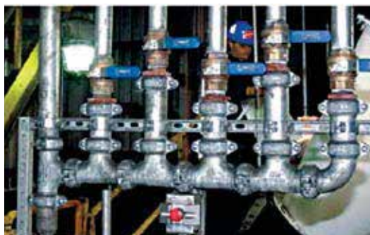
Custom control stations
