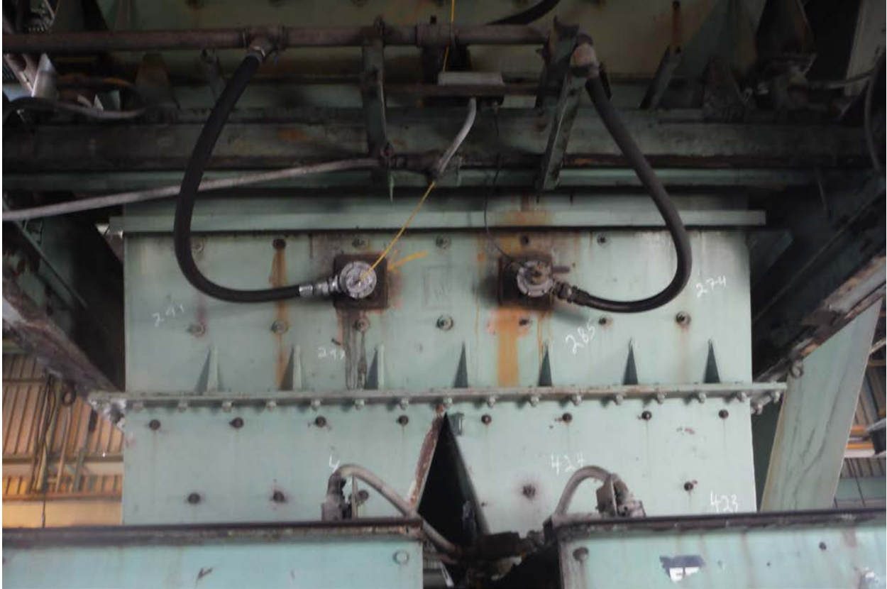
Clean Sweep nozzles Installed in Hopper Discharge: Note location of pilot box
