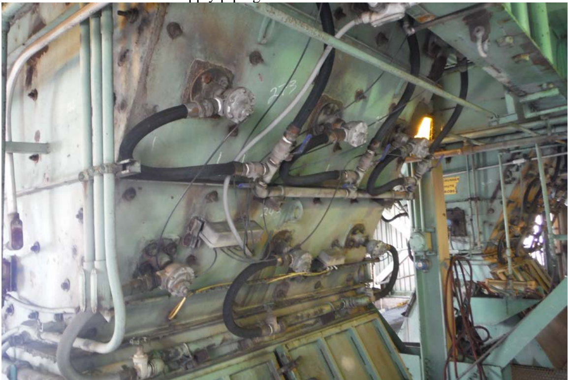
Clean Sweep Nozzles Installed in Chute to Remove/prevent Pluggage
