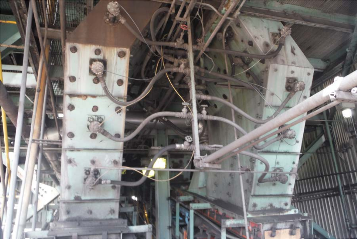
Note air supply piping installation with block valves
