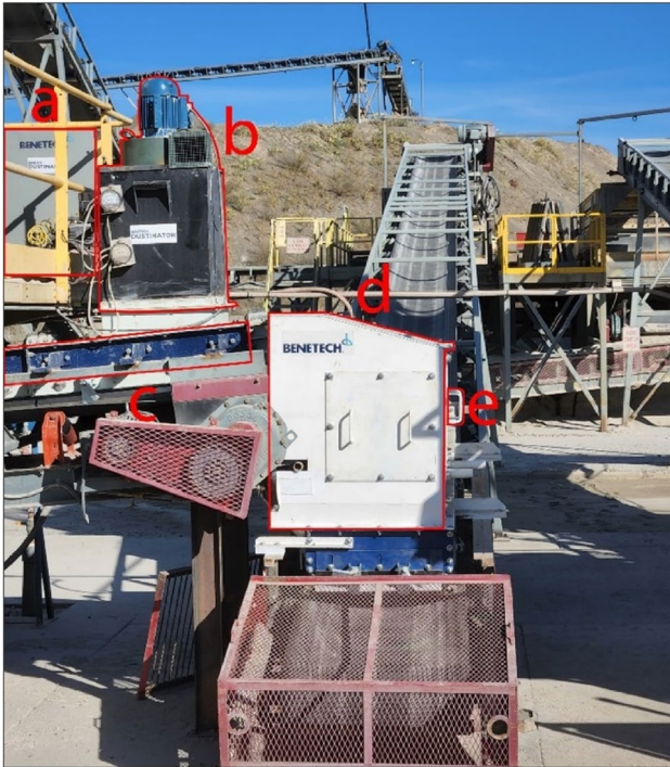
Fig. 7 Crusher/conveyor system at the CPM site, after installation of the dust control system: (a) MiniPak cabinet, (b) Dustinator, (c) shrouding/belt sealing system, (d) transfer point enclosure, (e) spray bar (at exit)
