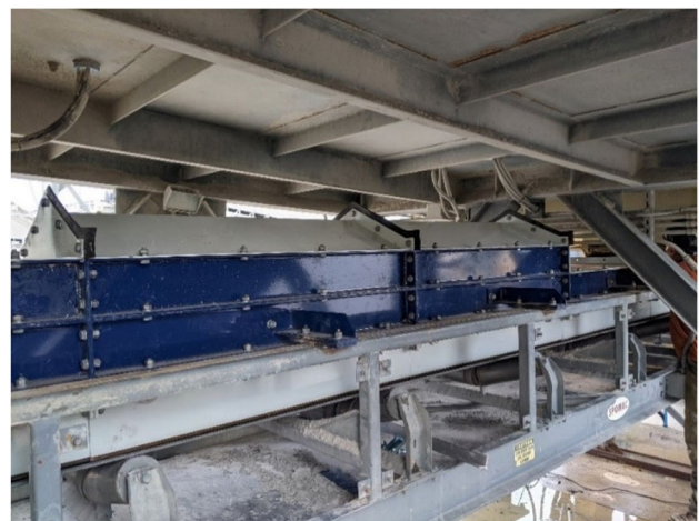
Fig. 1 Passive dust reduction system tailored to the #15 conveyor at CPM, based on Benetech®'s MaxZone® technology. The system comprises shrouds in sections with baffles at each junction, and a patented belt sealing interface with “XN liners” and dual-rubber adjustable seal
